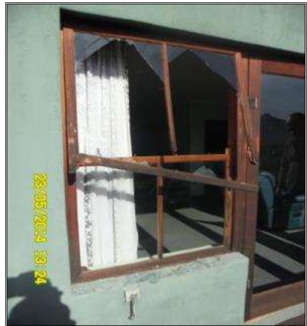
Fig.13. Window broken by DG6 in Bali Close, Capri. (May 2014)
