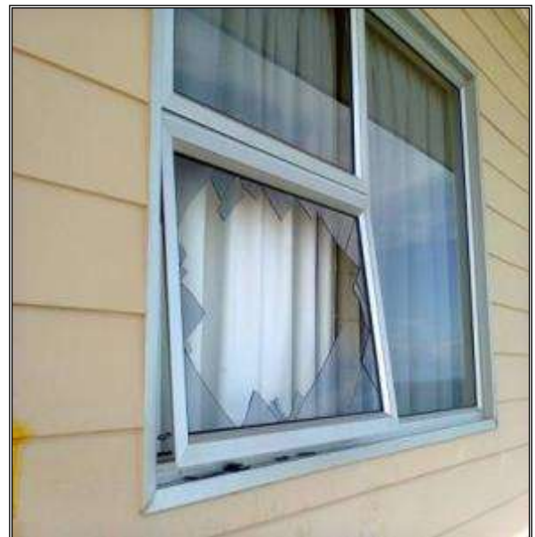
Fig.10. Window pane broken by GOB8 in Old Camp Rd.
